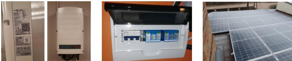
Fig. 2.12. Photographic documentation of the installed micro-generator (Sadales Tīkls, 2020)
